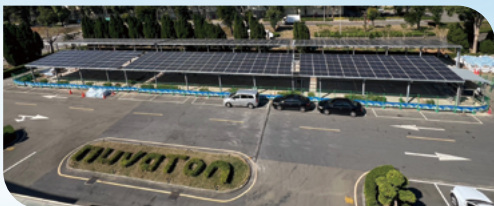
▲ Expansion of solar panels in the parking lot of the Yanshin Plant
